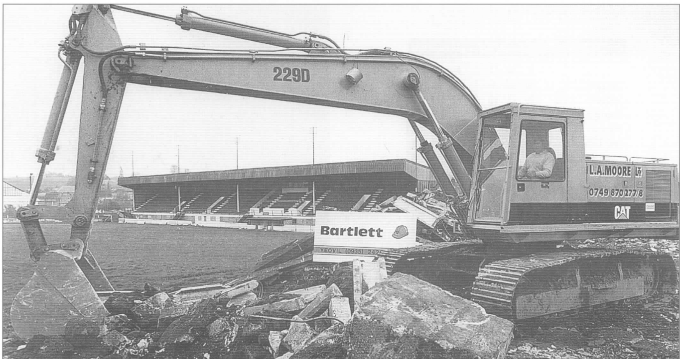
70 years of history disappeared in just a few days when demolition started.
